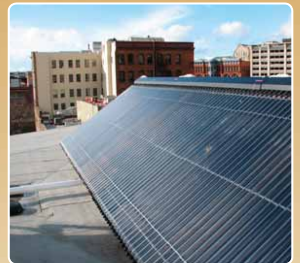
solar hot water heating panel arrays
